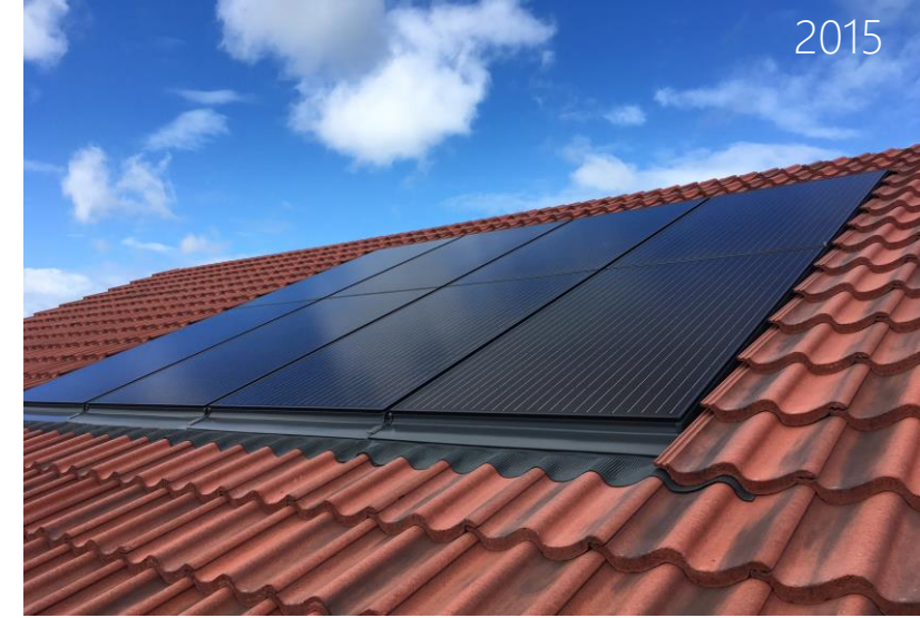
Clearline fusion Roof integrated solar photovoltaic panels
