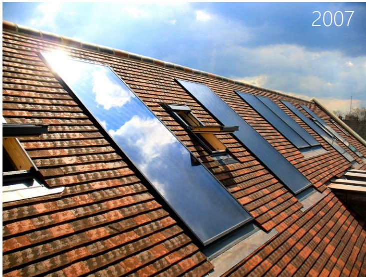
Clearline Roof integrated solar thermal panels
